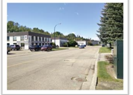
Missing sidewalks along 45 St
