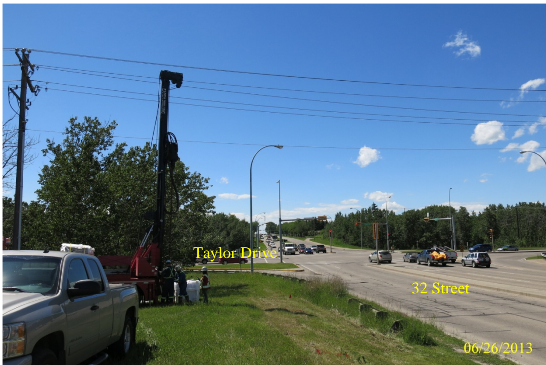
Photograph No. 6: Drilling MW-01 and VW-01 in northwest corner of the site. Note intersection of 32 Street and Taylor Drive in the background.
