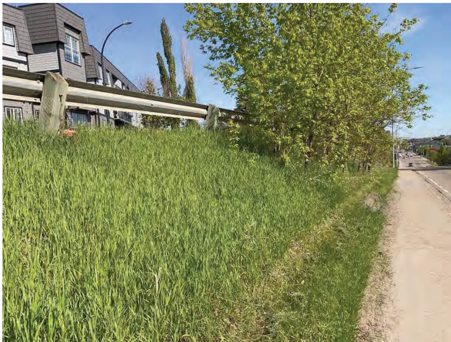
Photo 8: Slope near mid-section of embankment with leaning guardrail posts. Facing north.
