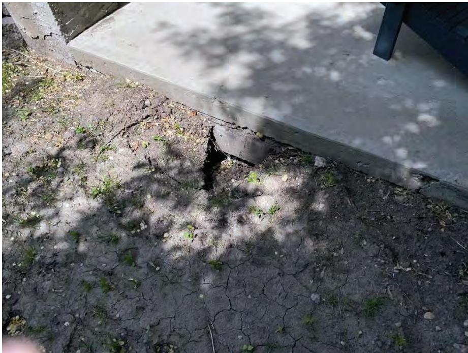
Photo 4: Hole in ground adjacent to far east unit patio slab at east building. Looking northwest.
