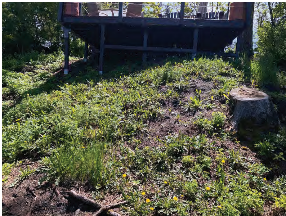
Photo 6: Soft, moist ground around deck structure on slope at Lot 14. Looking south (upslope).
