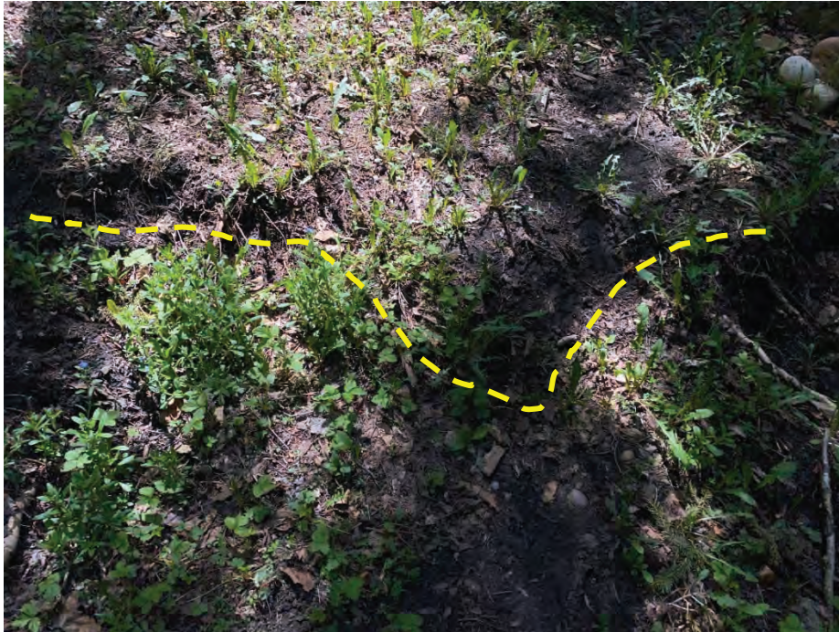
Photo 9: Open cracks in landslide mass, looking south.
