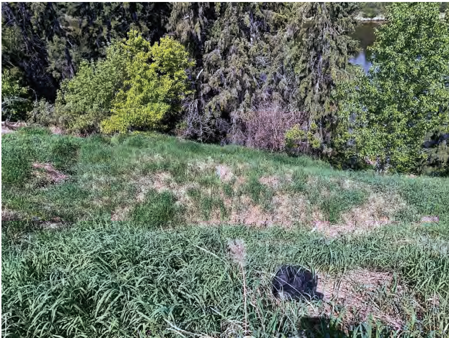
Photo 18: Landslide at east end of Warwick Drive, looking down slope.
