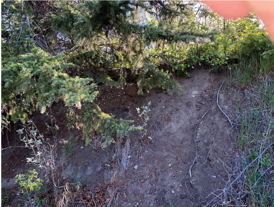
Photo 5: Exposed scarp face on historical failure north of the Kerry Wood entrance. Looking east.
