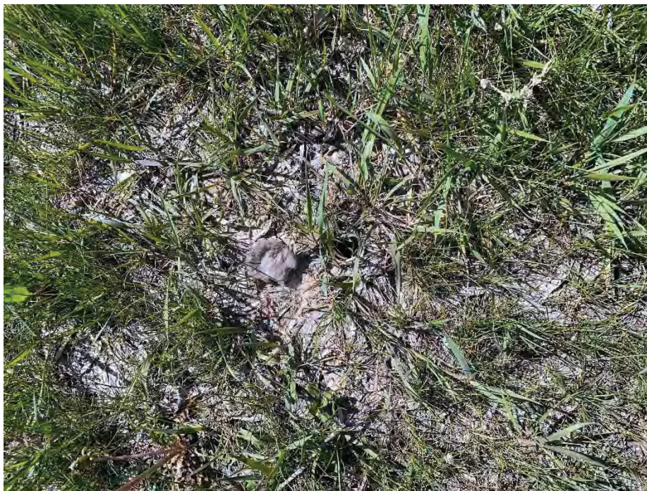
Photo 6: Damaged BH2 standpipe.
