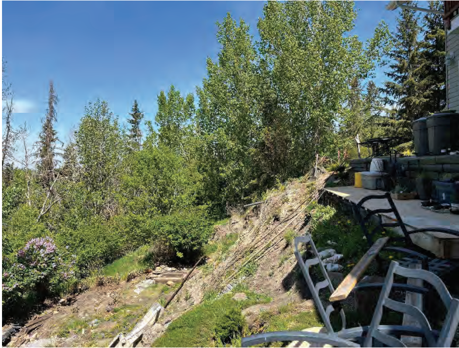
Photo 5: Backscarp encroaching the patio, facing north.
