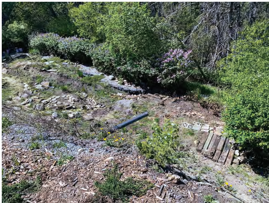
Photo 8: Exposed pipe at crest. Looking down to slide mass from north side of house, facing southwest.
