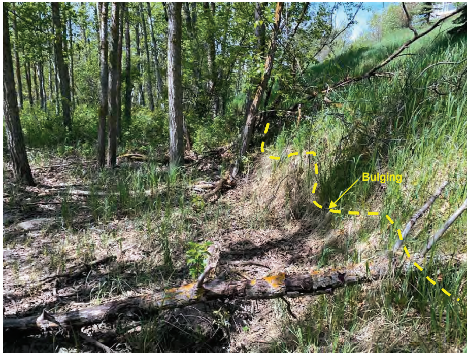
Photo 9: Toe of south slope with angled trees and bulging. Looking west.
