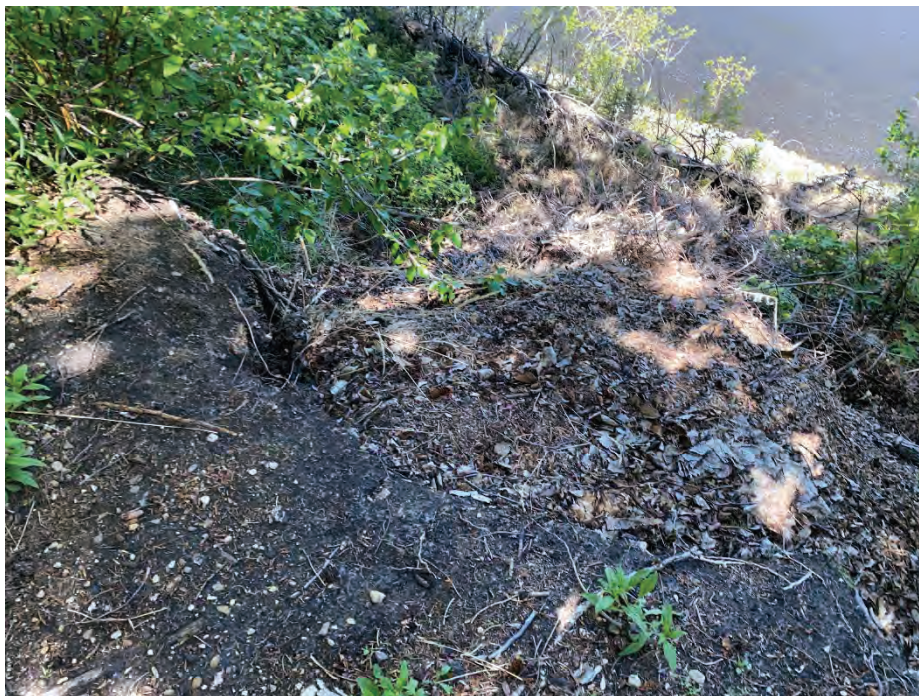
Photo 4: Soft, spongy ground at crest behind Lot 10, and accumulation of discarded brush on slope. Facing northeast.
