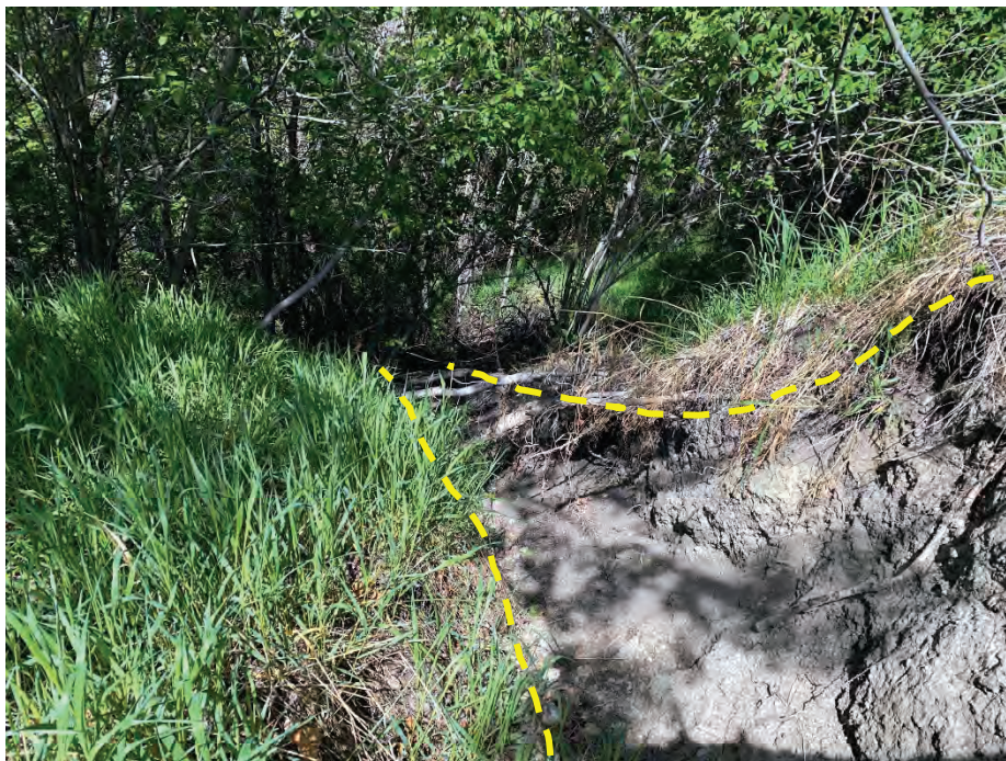
Photo 10: Erosion channel on north end of scarp, heading downslope. Looking northwest.
