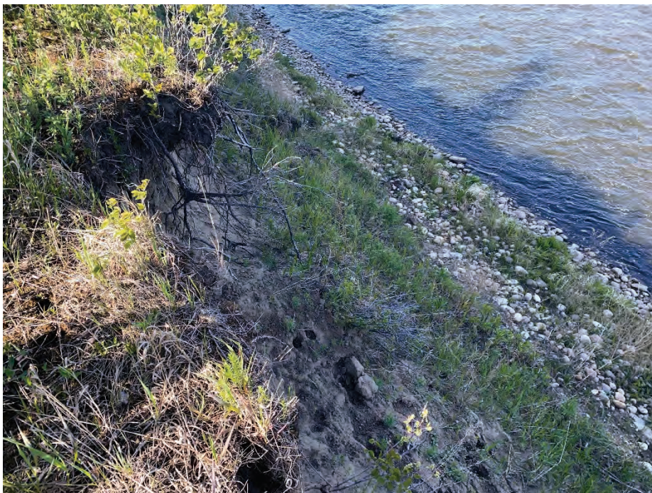
Photo 10: Undermining at edge of crest. Facing southwest.
