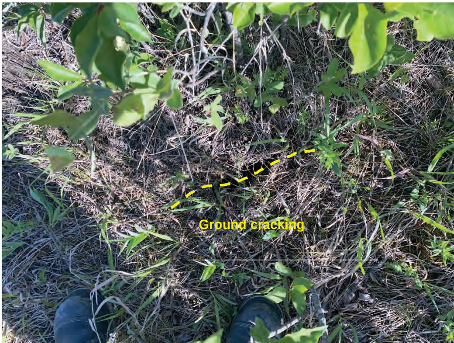
Photo 6: Ground crack near historical failure, 1.5 m away from crest. Facing north.
