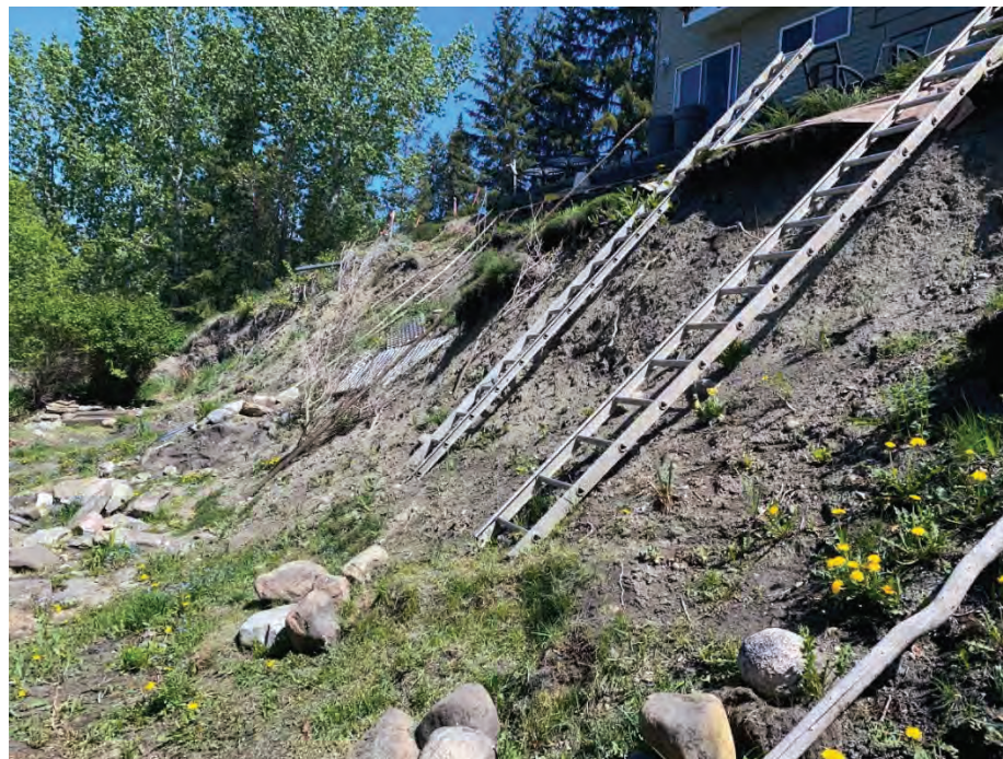
Photo 6: Exposed soil at backscarp. Lightly vegetated, at less of an angle. Facing northeast.
