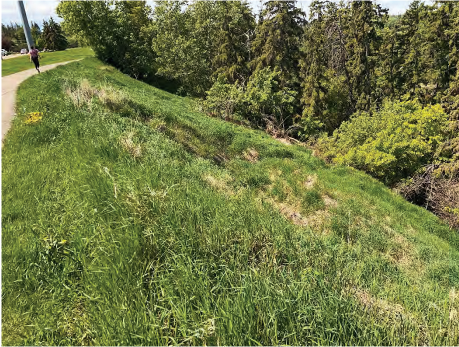
Photo 17: Slide at east end of Warwick Drive near recreational trail. Facing southwest.
