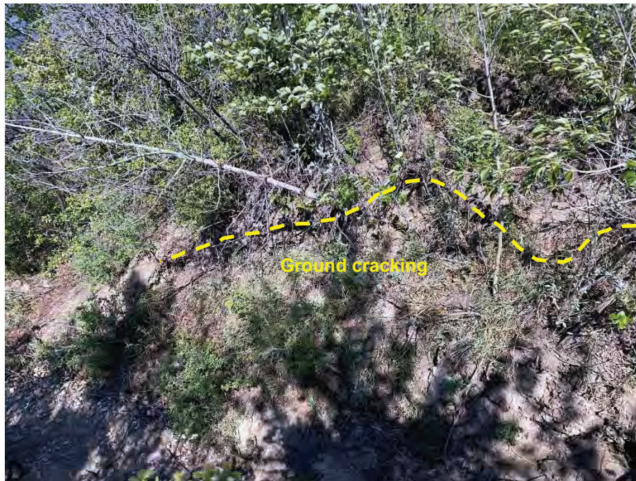
Photo 5: Slope failure at northeast end with ground cracking near crest. Facing northeast.
