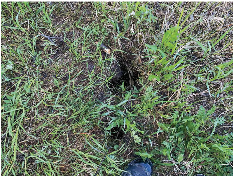
Photo 4: Gopher holes near north end of riverbank. Looking southwest.
