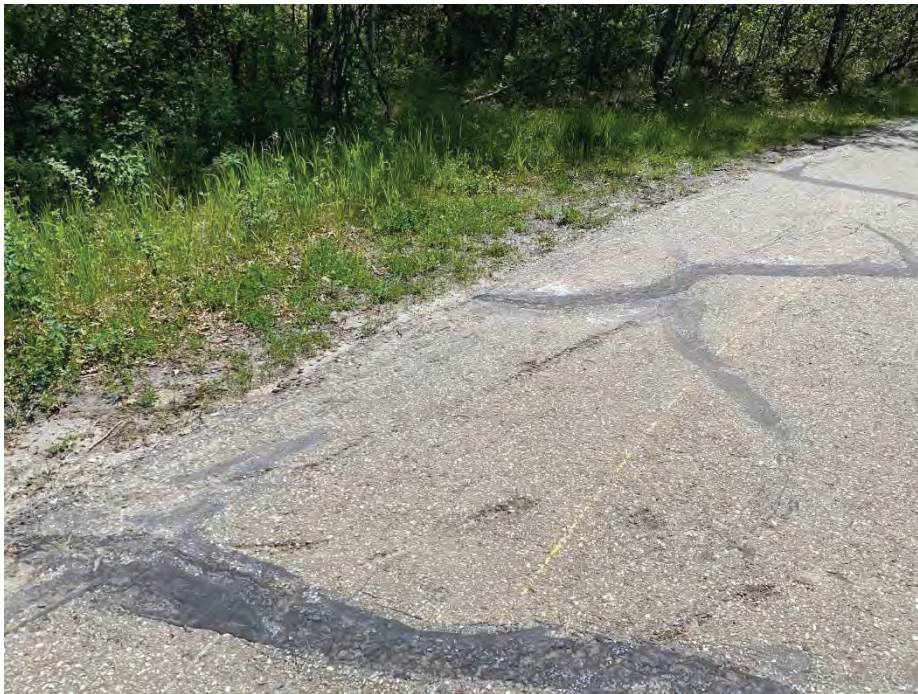
Photo 12: Creek pedestrian trail with some sealed and some open cracks. Looking south.
