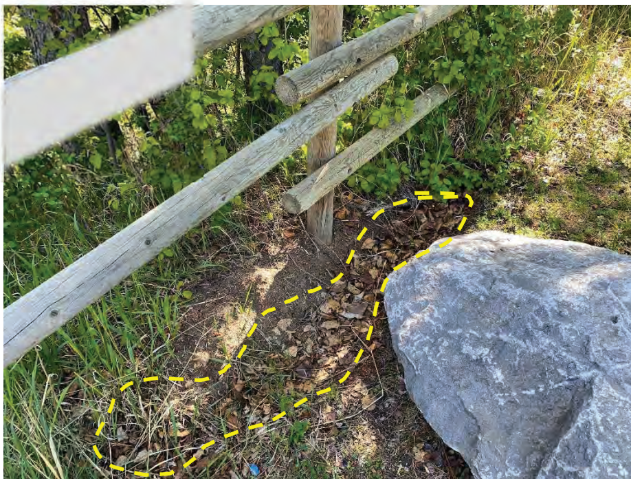
Photo 4: Ground crack near trail fence midway up embankment. Facing east.
