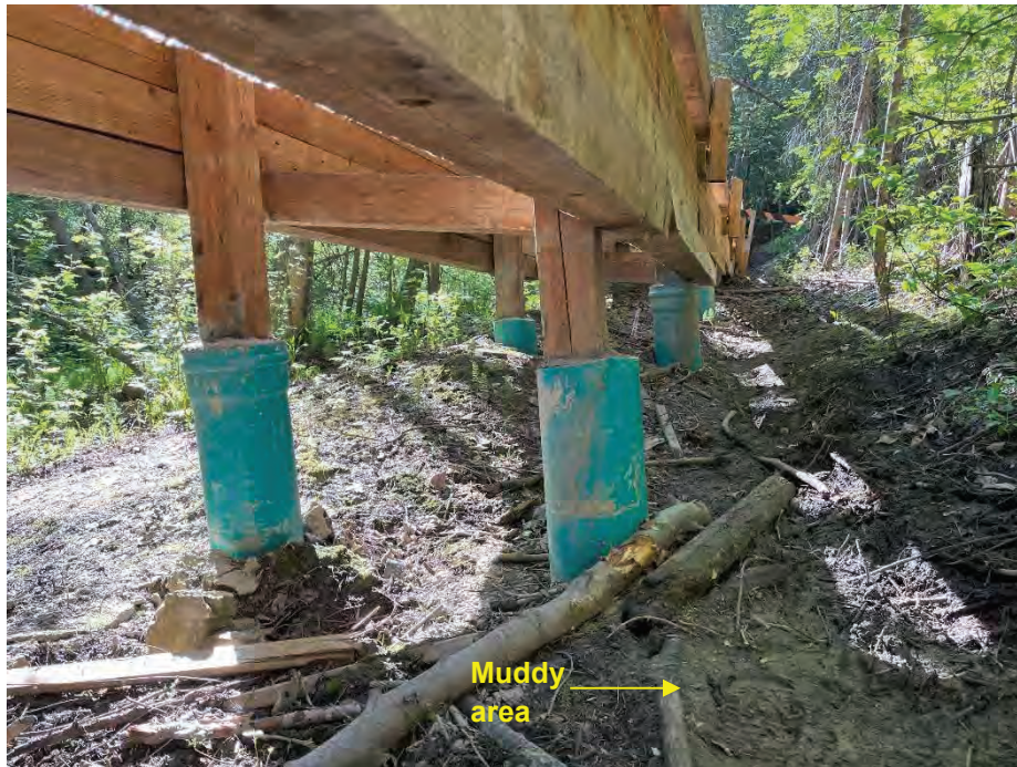
Photo 3: Damaged section of wooden walkway north of 4806 36 th Street. Looking southeast.
