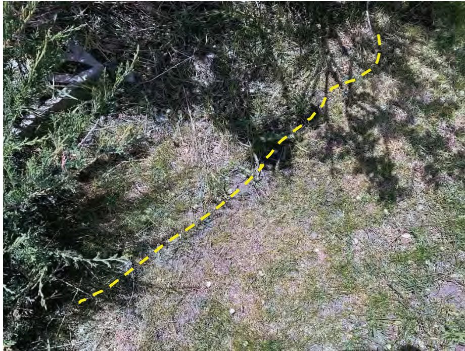
Photo 7: Old ground crack on south slope. Looking northeast.
