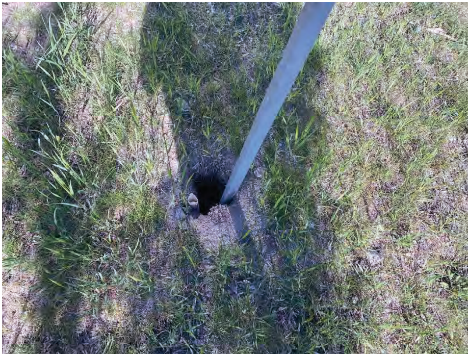
Photo 12: Hole with stake and broken PVC standpipe east of former Elks building. Facing south.
