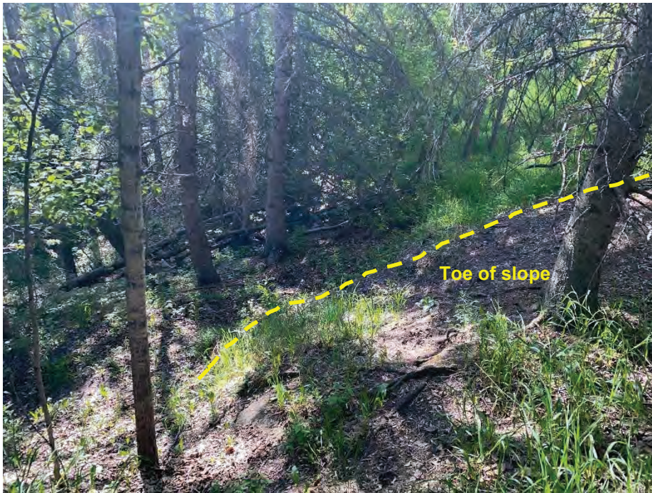
Photo 14: Historical failure northeast of former Elks building. Facing west.
