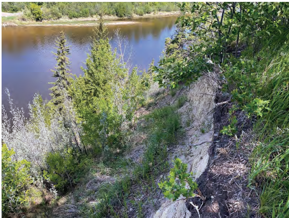
Photo 16: Slide at recreational trail lookout on Warwick Drive, facing northeast.
