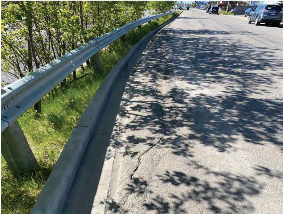
Photo 3: Cracks and surface depression on Gaetz Ave Service Road. Facing south.
