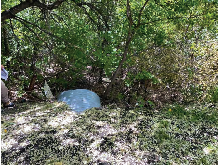
Photo 5: Culvert draining onto south slope. Looking south.
