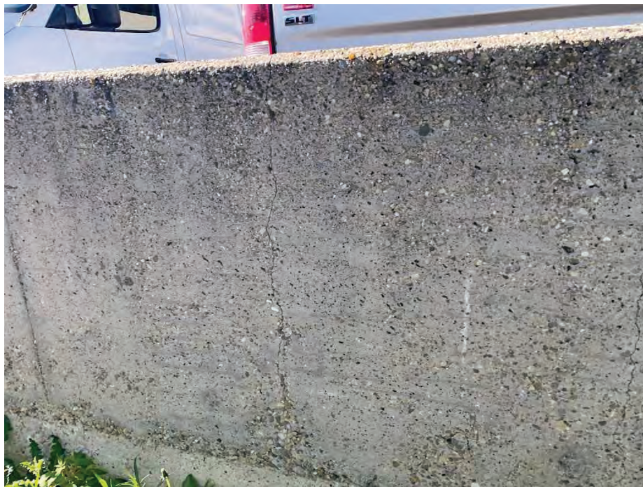
Photo 10: Hairline cracks in concrete parking wall of the apartment complex. Facing southwest.
