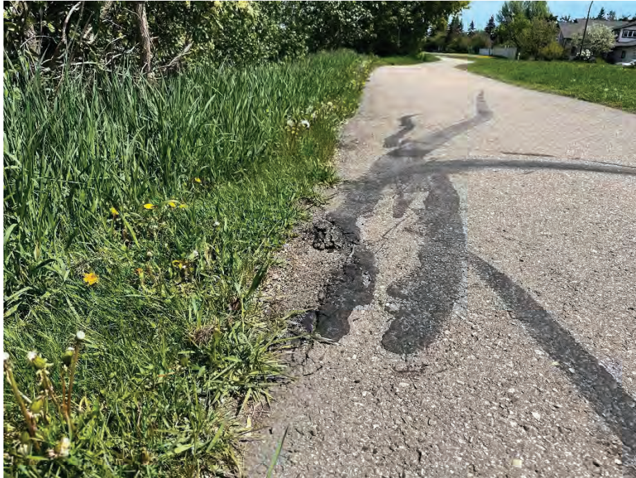
Photo 19: Cracking and heaving on edge of asphalt trail at east end of Warwick Drive. Looking east.
