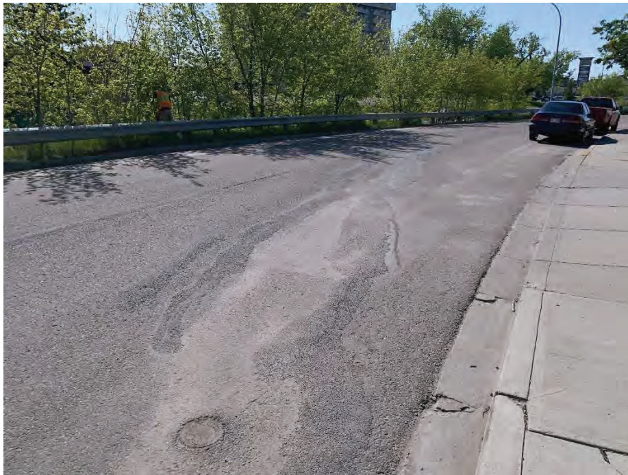
Photo 4: Sealed cracks by the apartment entrance.
