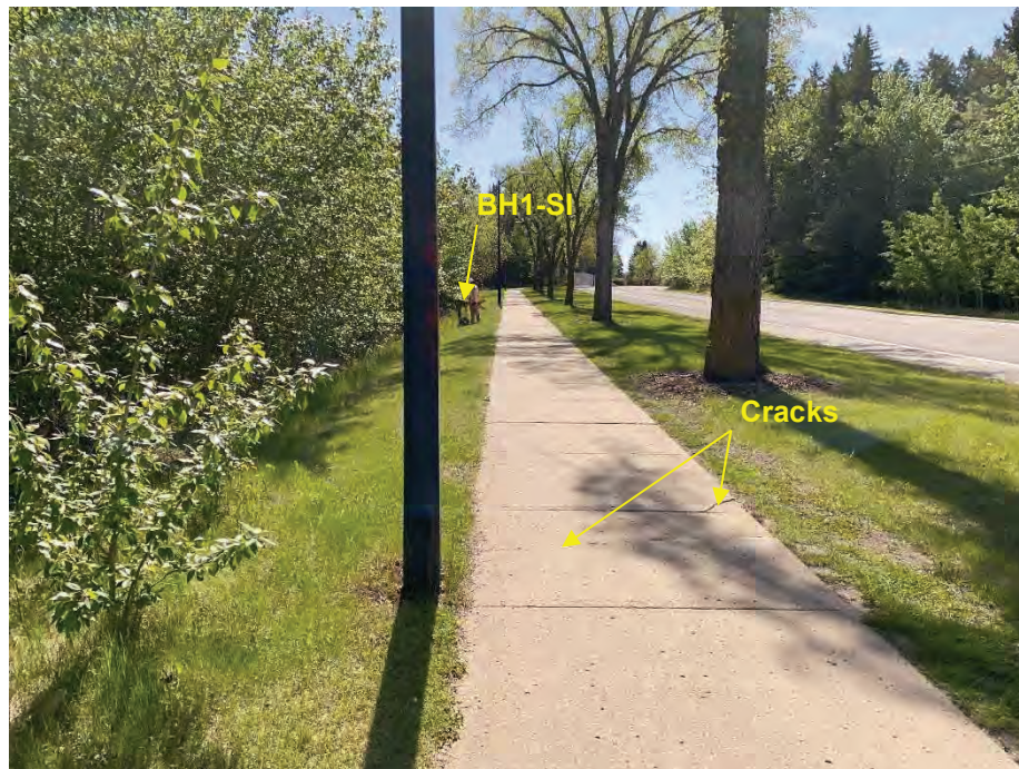
Photo 2: Sidewalk cracking above the embankment area. Facing east.
