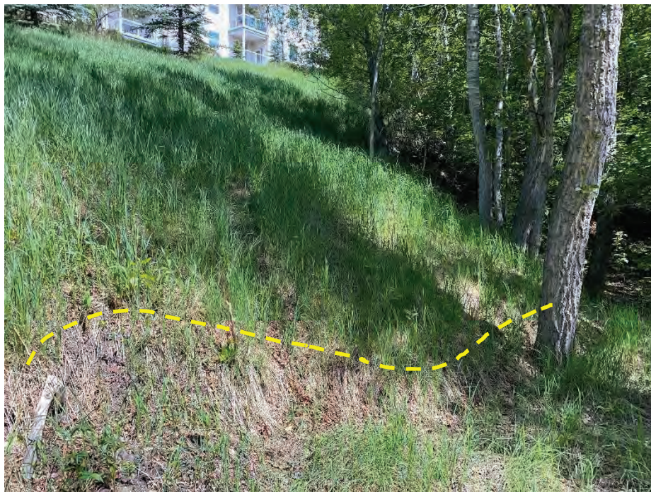
Photo 10: Toe bulge at south slope. Looking north.
