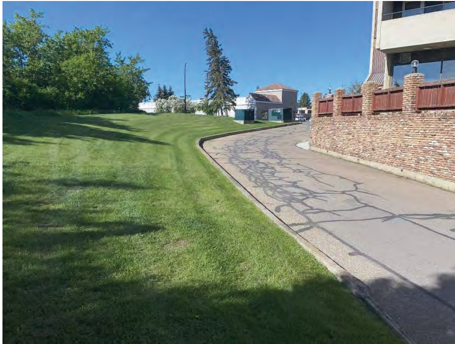
Photo 7: Access road east of apartment complex with sealed cracks. Facing southwest.
