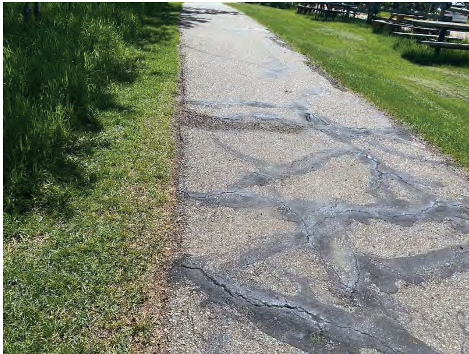
Photo 4: Sealed cracks in asphalt pedestrian trail, looking southeast.
