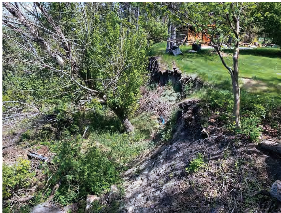
Photo 10: Scarp of landslide behind Lot 18. Facing east.
