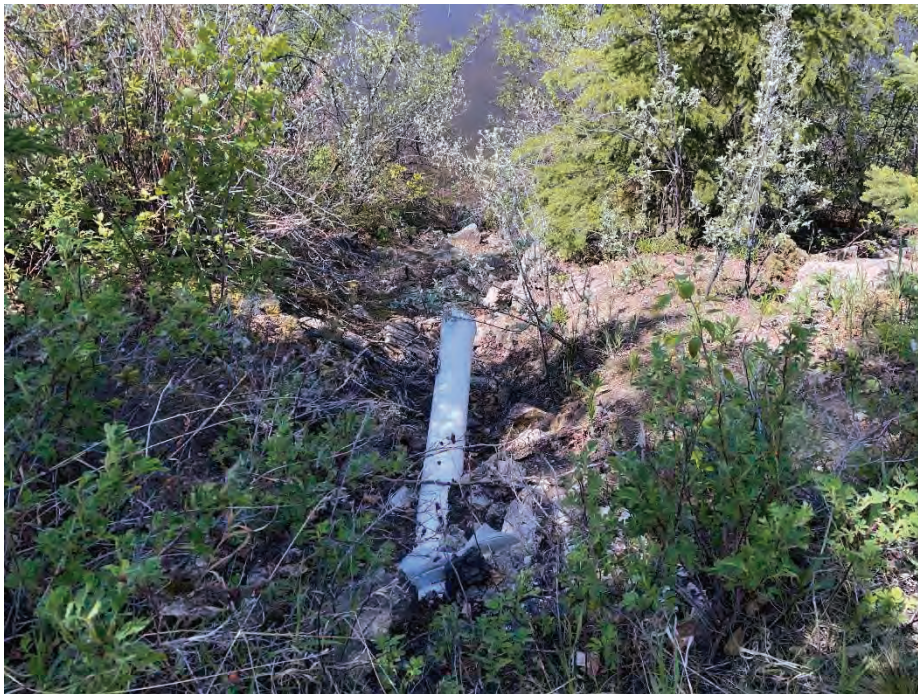
Photo 2: Northeast outfall directing into 150 mm PVC pipe. Erosion channel is approximately 1-2 m wide below the outlet. Looking west.
