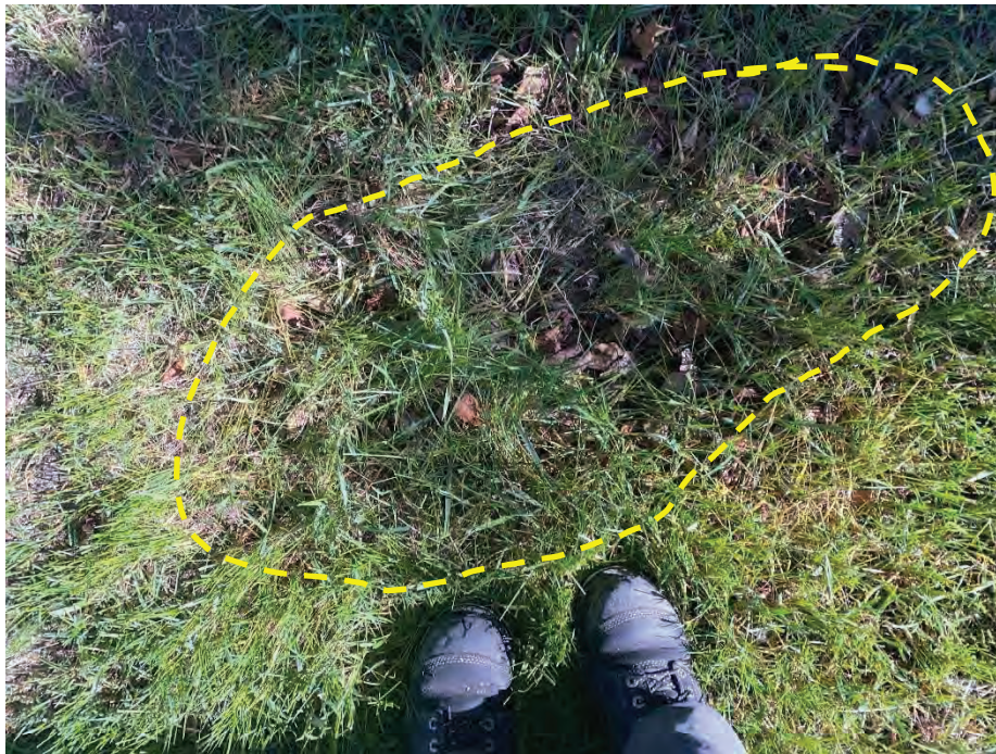
Photo 4: Ground depression northeast of Lot 4. Facing north.
