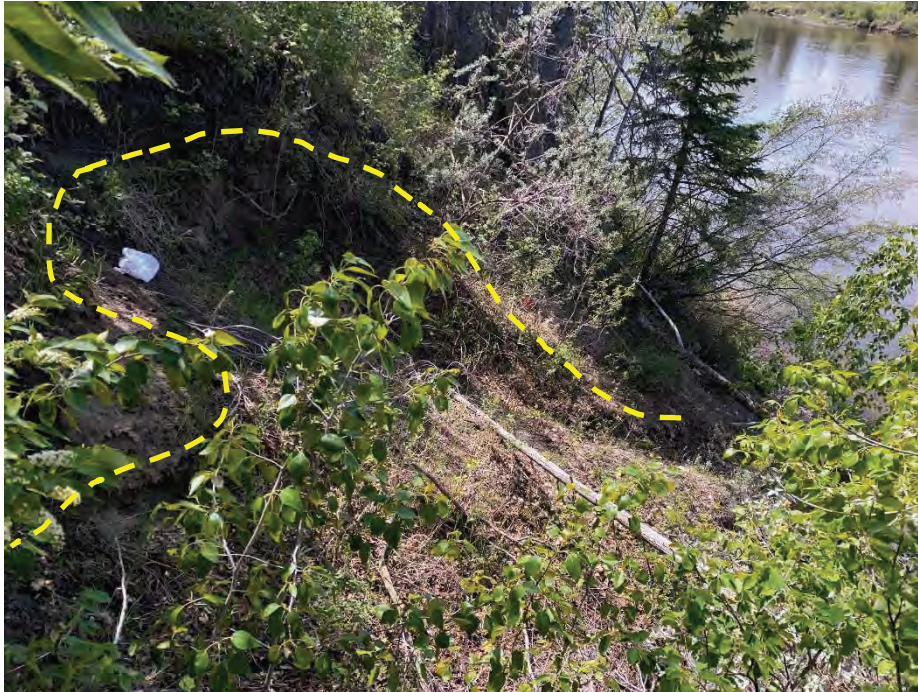
Photo 3: Northeast historical failure. Looking north.
