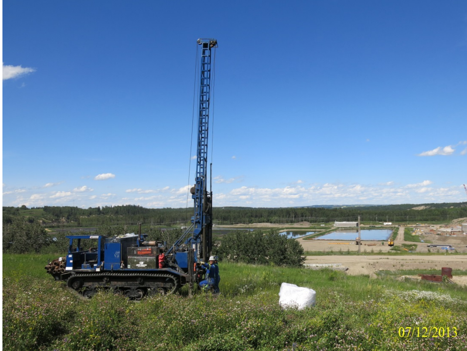
Photograph No. 11: View of drill rig at location of TH-06, looking north.
